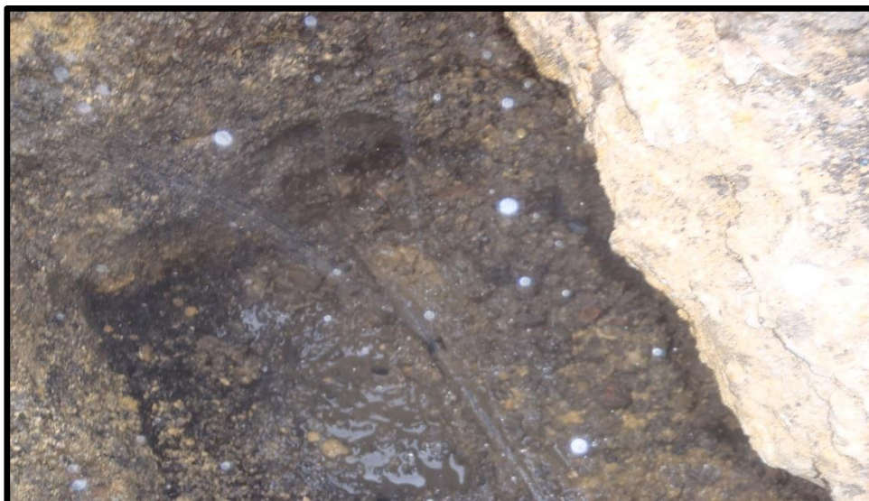
Picture 3 – The leak on the 20mm supply pipe
