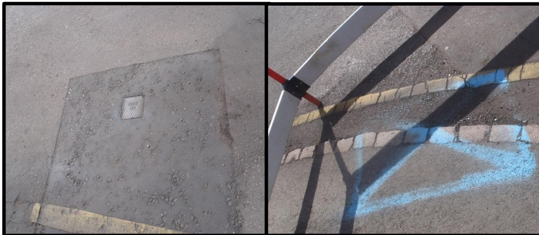
Picture 1 – Water Meter Location
