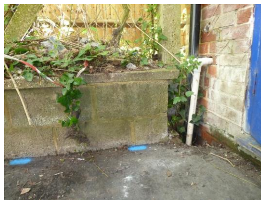
External line of pipework up to building
