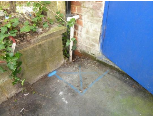
Location for trial hole to locate pipe and prove leak is under the building
