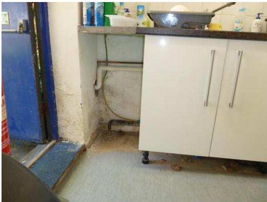
Rising main in kitchen area of the Ceramic Tile Distributors
