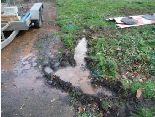
Leak rising through ground
