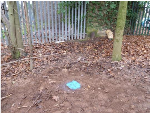
New isolation valve outside substation
