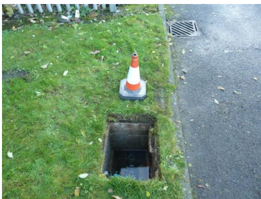
Leak location behind water meter (traffic cone)
