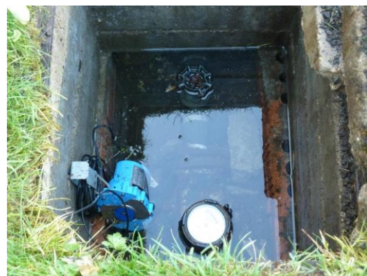
Water in chamber (level drops when gate valve closed)
