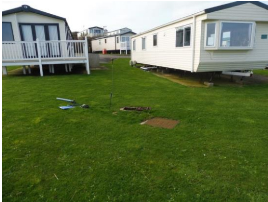
Location of leak on isolation valve between 5/6 Bramp Heights
