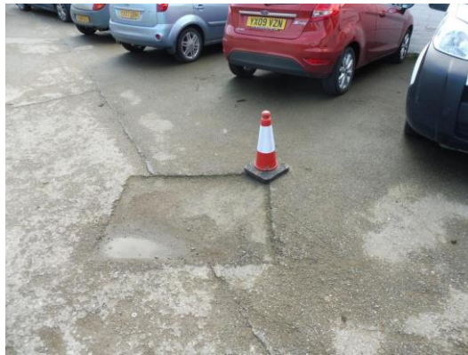
Leak 1 - location marked by traffic cone
