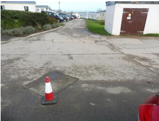
Leak 1 - location in staff parking area
