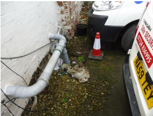
Leak to excavate by staff canteen – high leak noise
