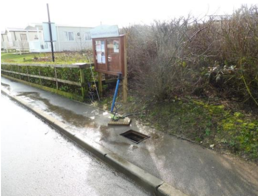
Location of leaking Fire Hydrant
