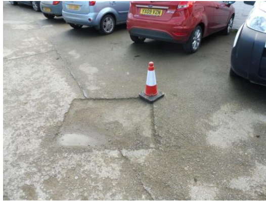
Leak 1 - location marked by traffic cone
