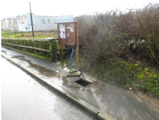
Location of leaking Fire Hydrant
