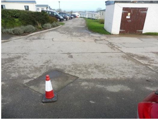
Leak 1 - location in staff parking area
