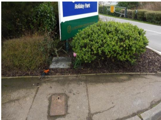
Second meter location
