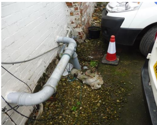
Leak to excavate by staff canteen – high leak noise
