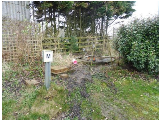
Main meter location
