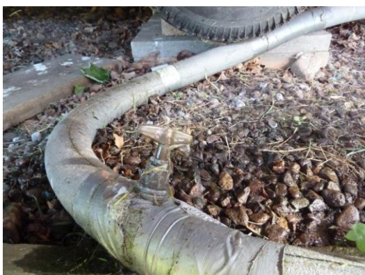
Leak on stoptap – plot 69 Morpeth Mews
