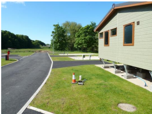
Leaking stoptap supplying new Woodside development
