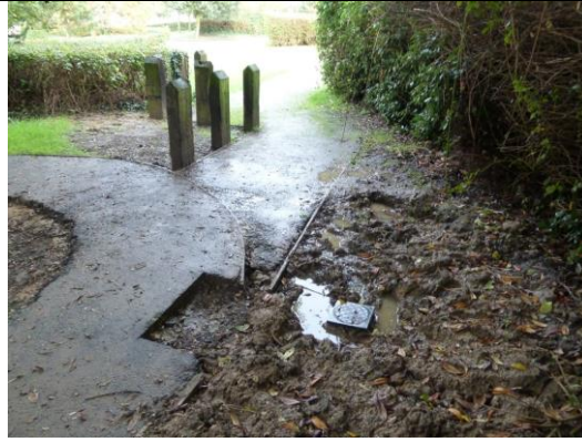
Leak location 4 – leak on pipework by new atlas box
