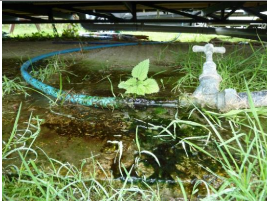
Leak on stop tap - 42 Meadowside
