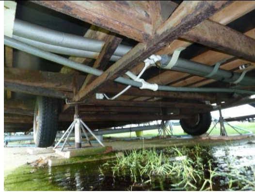
Leak on drain cock – 77 Hillside Drive
