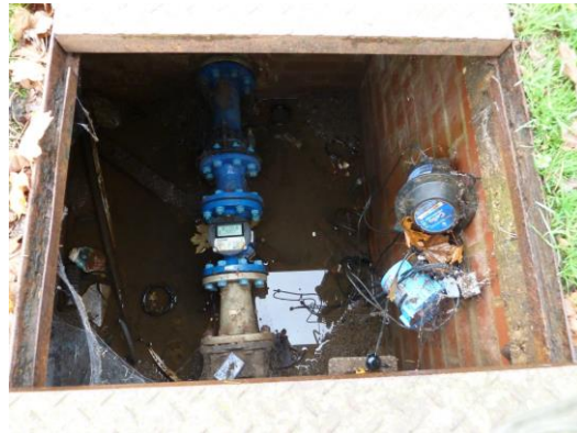
Meter chamber and water flow data logger
