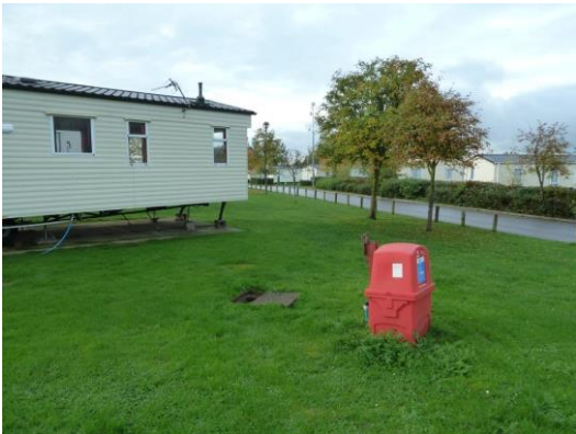
Leak location 5 – leak on below ground pipe [Unable to pinpoint without tracing pipework out]
