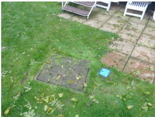
Leak location 1 – leaking stoptap by 15 Sidings
