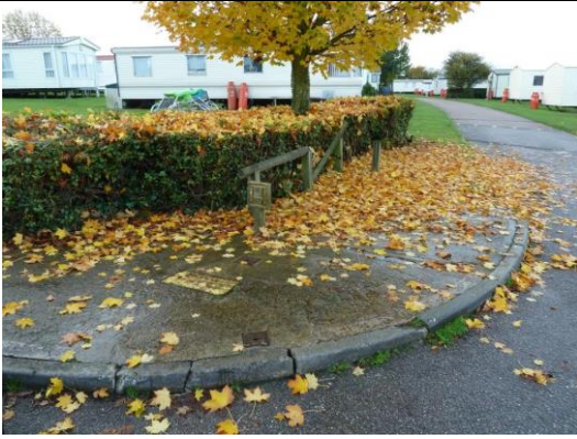
Leak location 3 – Fire Hydrant valve passing
