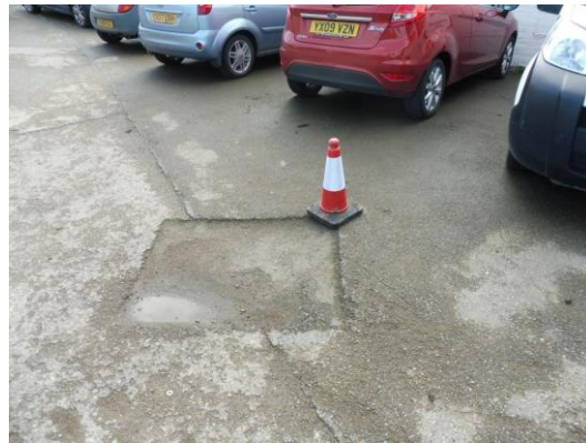
Leak 1 - location marked by traffic cone
