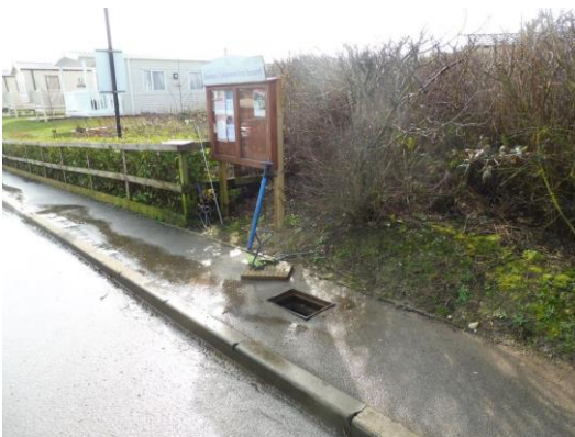
Location of leaking Fire Hydrant
