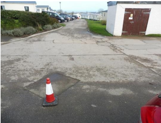
Leak 1 - location in staff parking area
