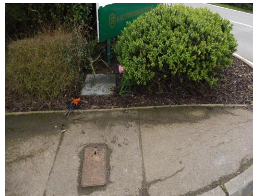
Second meter location
